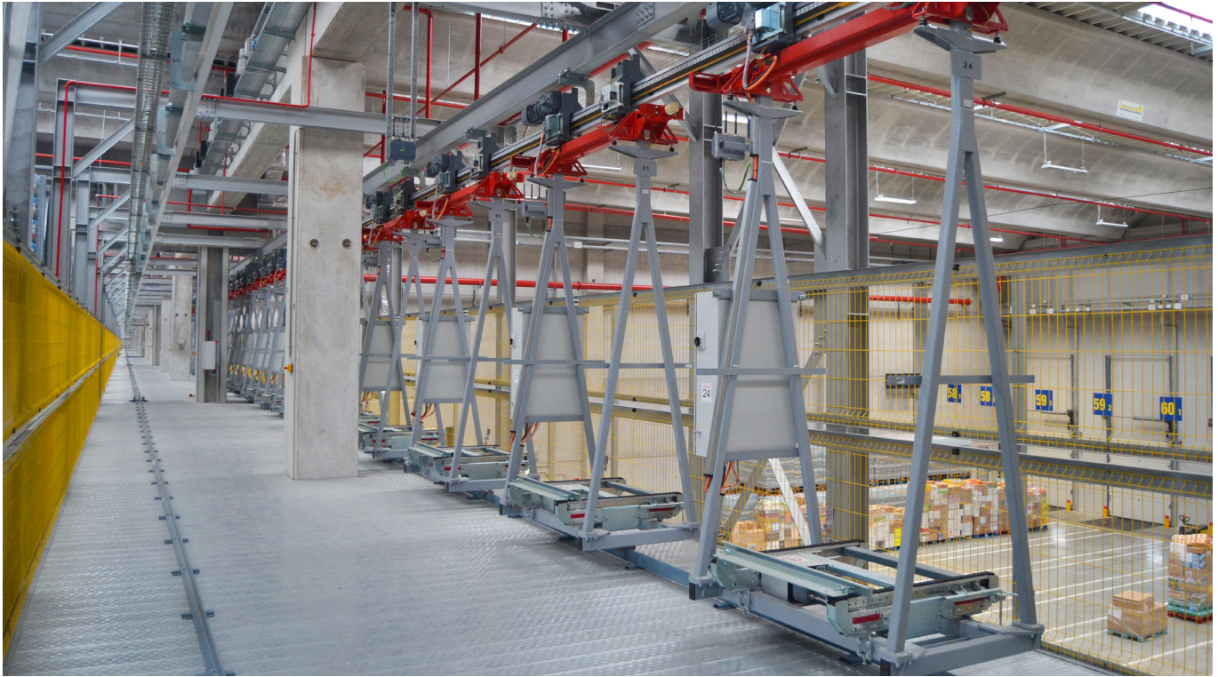
A monorail suspension system conveys the pallets within the extended Almarai production complex. 40 monorail trolleys are in use in the logistics center alone.
