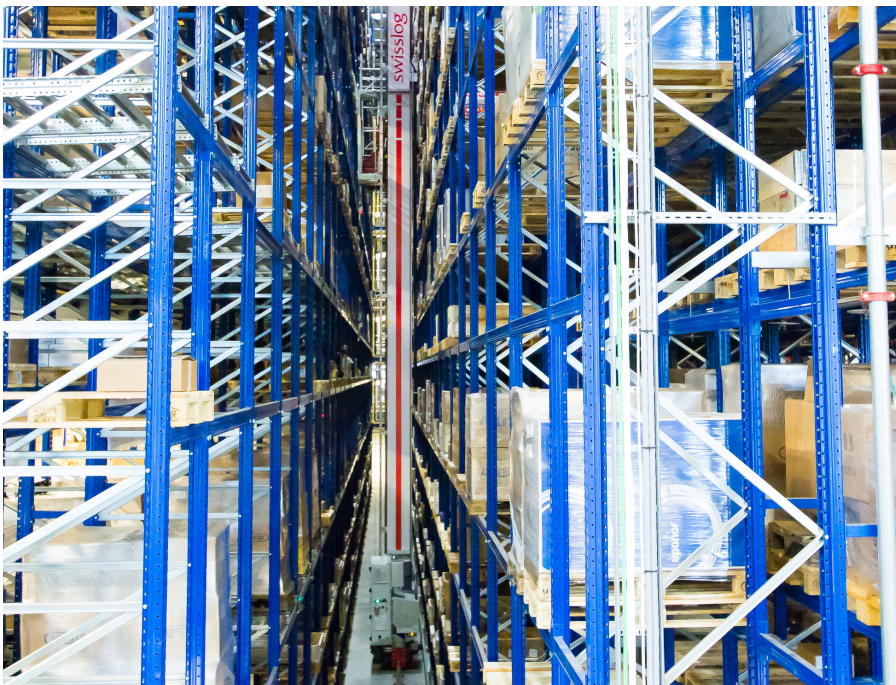
The Vectura automated storage and retrieval stacker crane from Swisslog provides reliable handling of pallets in the Almarai high-bay warehouse.
