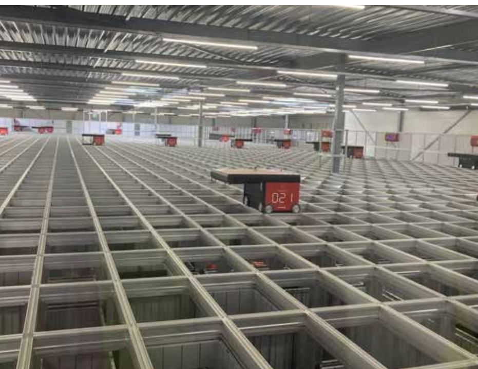
The AutoStore has a storage capacity of 29,000 totes.
