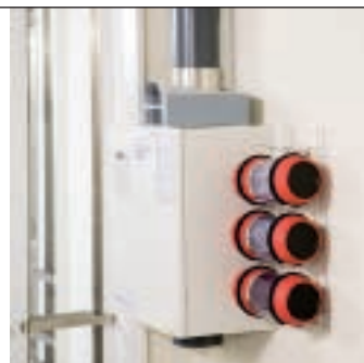
Pneumatic tube system station with storage function
