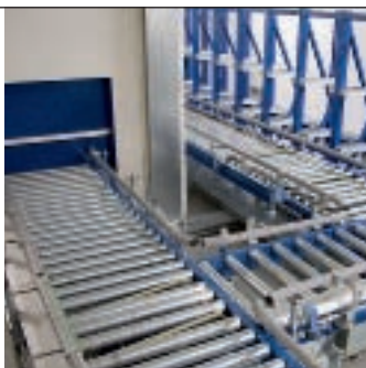
Containers ordered from the high-bay warehouse in the vault are carried by an automatic conveyor system to the elevator ...
