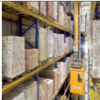
Stacker cranes store the pallets in the high-bay warehouse
